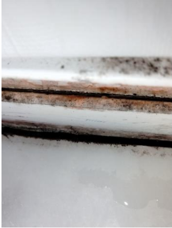
A wall with mold
